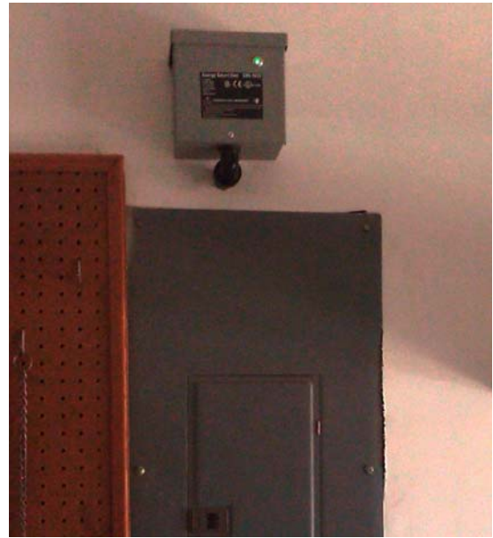
Picture 2 – Indoor above panel mount
